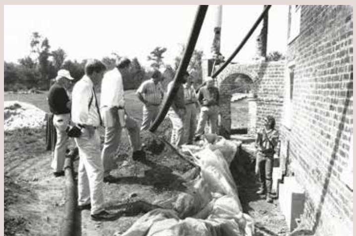
Outer brick walls underpinned with concrete footings and a drainage system during stabilization phase, 1993
