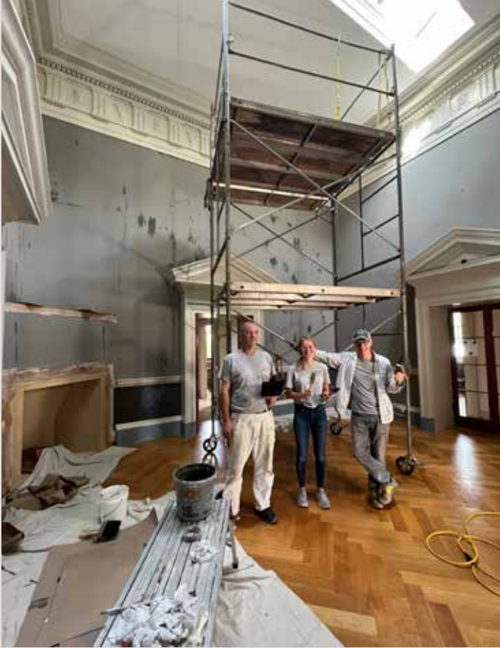
Historic Painters L-R: Brad Stewart, Ginna Stillwell, Chris Mills in the dining room after applying the historic distemper paint to the plaster walls, 2022
