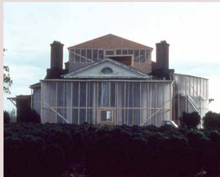
Enclosures around the house to allow for winter use of lime mortar; structure on top to allow for the removal of the 1846 roof, 1995
