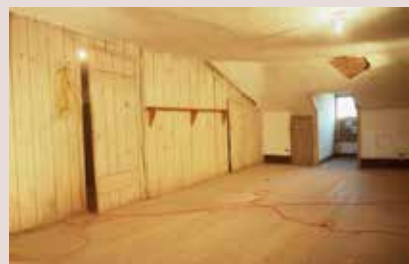
1846 attic inserted above the middle room which reduced the lower middle room from a 20' ceiling to a 12' ceiling, 1995
