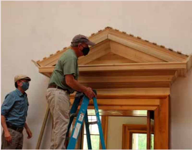
Craftsmen C. J. Frost and Dave Clauss install one of the six classical doorway pediments, 2022
