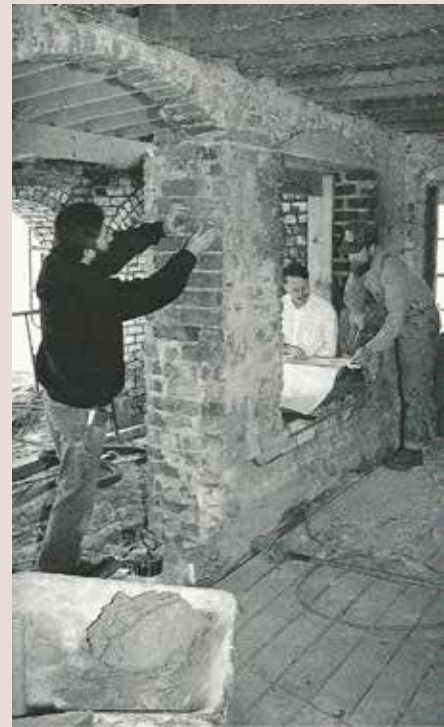
Investigation and brick repair on the lower level: L-R: Henry Cersley (mason), Travis McDonald, Douglas Rideout (restoration supervisor), 1995
